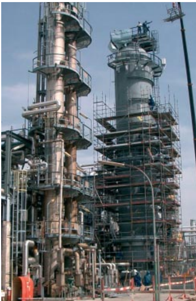
Fig. 8: Down-flow fixed-bed reactor for HDS, HDN and HDA diesel treatment (right).
